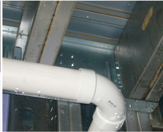
Wall-panel Prefab used building information models to eliminate conflicts with the MEP trades.
