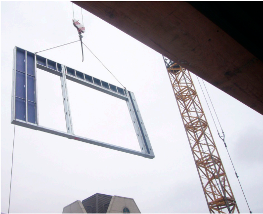
Wall-panel prefabricated the wall and floor panels off site. Wall-tech erected the systems.
