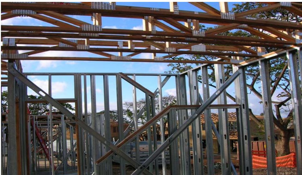
Floor joists supported by steel wall panels. Note that the trusses are each directly located over a stud (inline framing). Further, in order to avoid unusual connection details between the floor trusses and the steel walls, a wood top plate is installed on the panels during fabrication at the panel plant.
